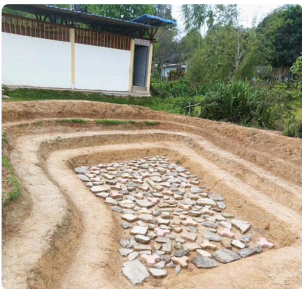
Experimental Rainwater Harvesting Pond
